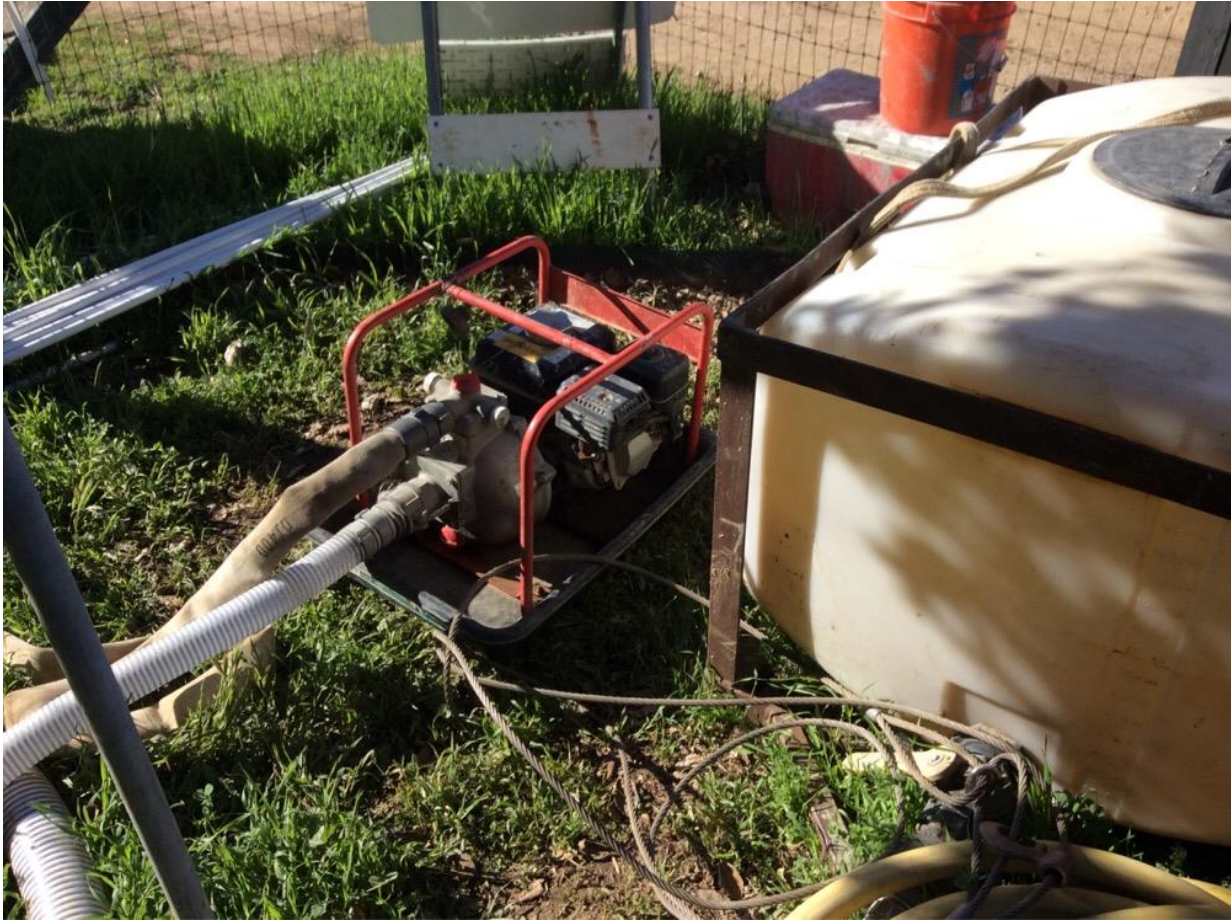
Photo 5: In accordance with MM PHS-2, a water pump at Pole Z118042 (TL 682) was staged in a drip pan to prevent any possible leaks from being discharged into the ground.
