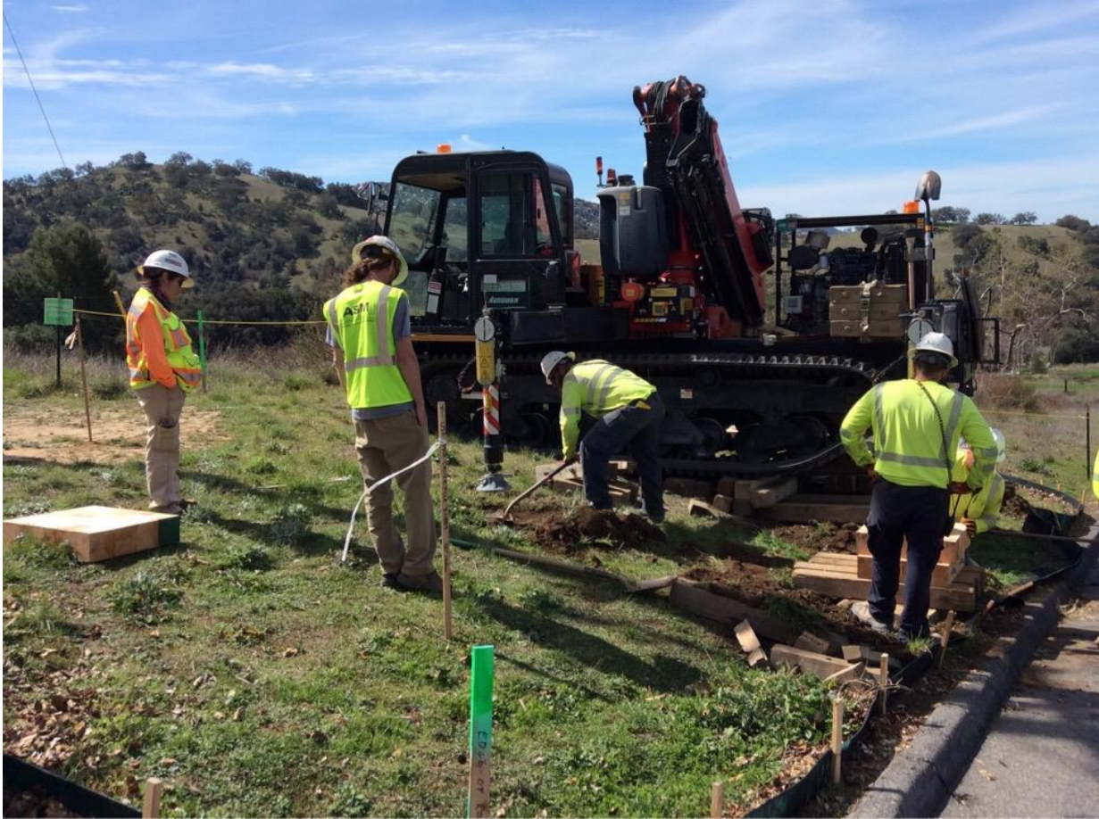
Photo 4: During site setup at along TL 682, ESA signage was present and cultural resource monitors were observed monitoring ground disturbance to level the ground for outriggers, in accordance with the Historic Properties Management Plan, MM CUL-1, MM CUL-3, and APM CUL-04.
