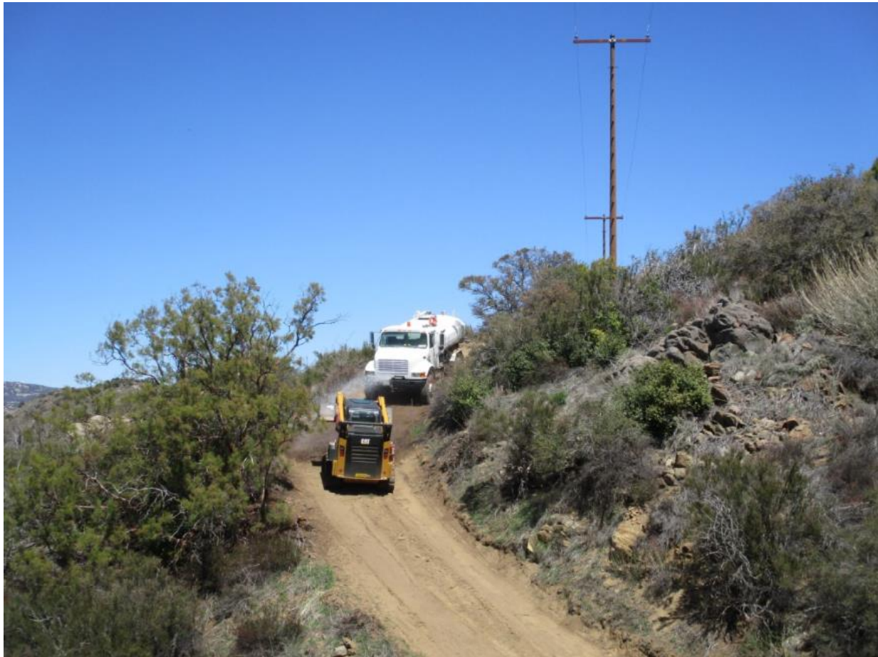
Photo 2: In accordance with APM AIR-02, a water tender was observed applying water during water bar construction at P176955 (C442).
