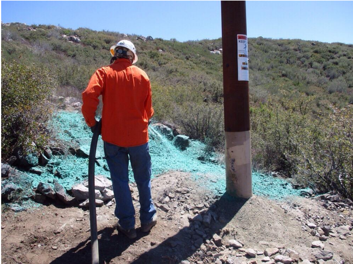
Photo 6: A construction worker was observed applying hydro-mulch at P258115 (C 442), in accordance with the Habitat Restoration Plan (MM BIO-4) and the Erosion Control Plan (MM HYD-1).
